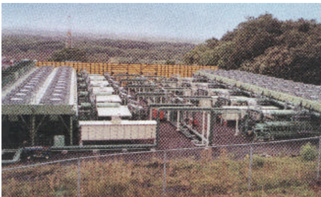
Figure 11. Puna Geothermal Venture Power Plant (Ormat, undated).
